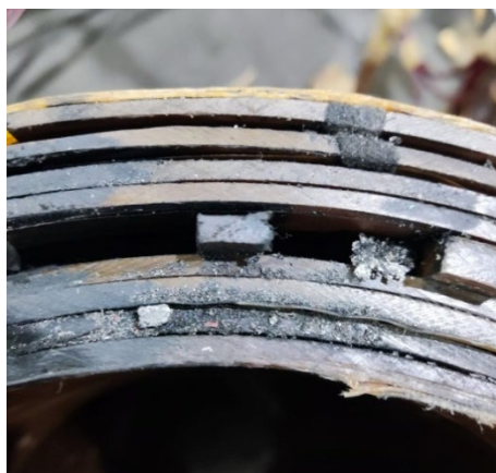
Figure 2 – Damage to the internal insulation of power transformer windings
